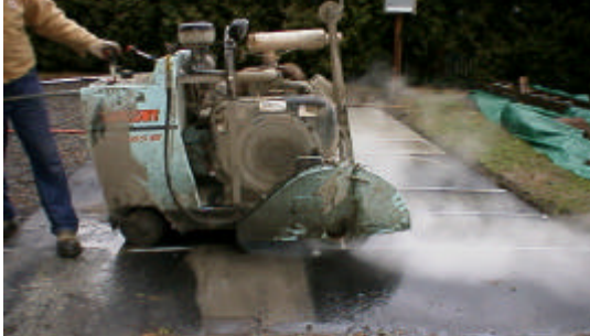
Figure 8. Cutting slots into the asphalt and concrete sections of the Blue Road Research test pads.
