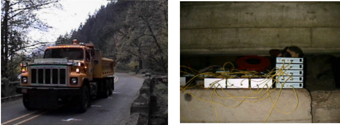
Figure 2. Test vehicle used to support static and dynamic testing of the Horsetail Falls bridge and five high speed, high sensitivity fiber grating demodulation systems deployed by Blue Road Research underneath the bridge for high speed measurements.
