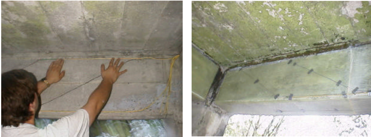
Fig. 6 Sensors being placed into grooves in the concrete (left) and embedded into the composite wrap (right)
