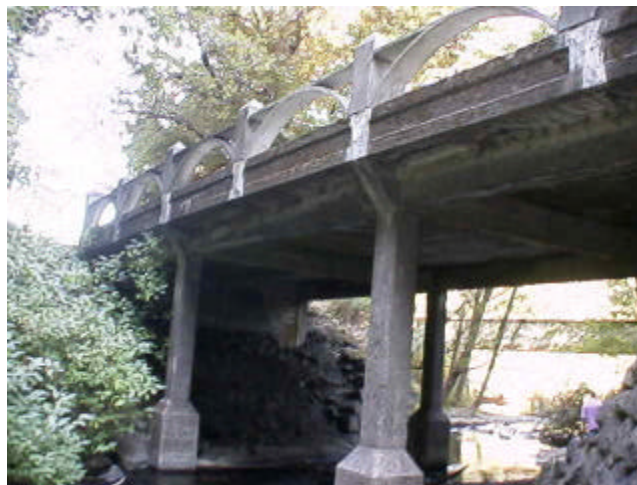
Fig. 5 Horsetail Falls Bridge before being strengthened by composite wrap and instrumented with 26 long gage fiber grating strain sensors
