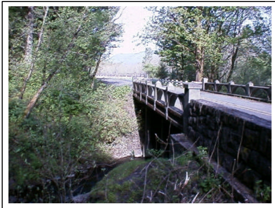
Figure 5. Horsetail Falls Bridge, Oregon, scheduled to be instrumented with fiber sensors in summer 1998.
